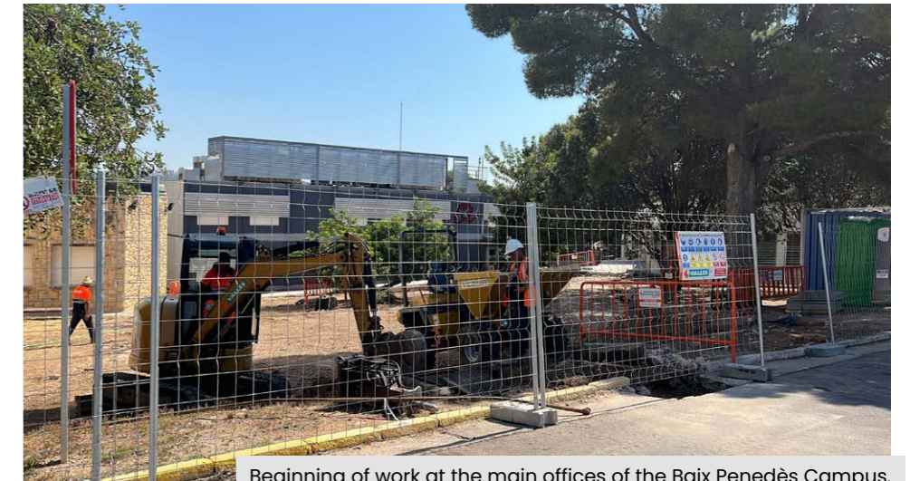
Beginning of work at the main offices of the Baix Penedès Campus.
