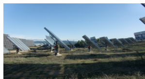
Vista general parc solar
